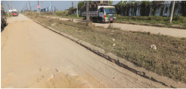
Poor road infrastructure is evident at many industrial estates
